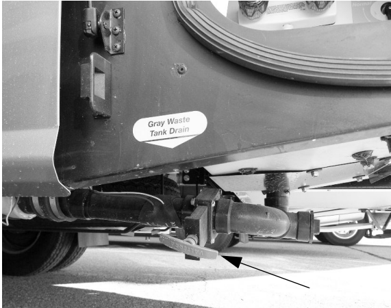
Gray Waste Tank Drain Valve (Located beneath rear driver side of the motorhome) -Typical View
