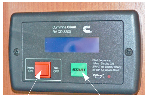
Diesel Generator Start/Stop Buttons (Located near monitor panel) -Typical View
